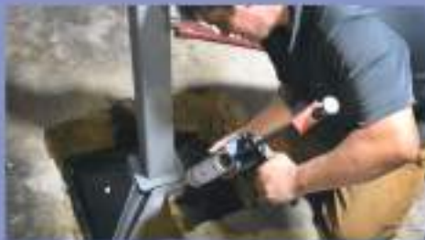
5. Inject poly urethane foam into injection ports located on footing to fill voids in soil creating a stable base.
